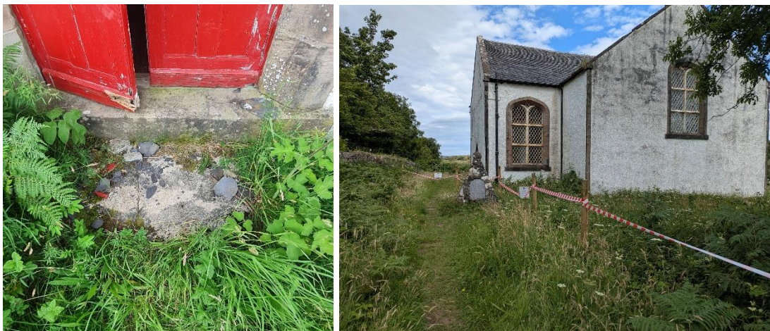
Two months later – photos taken in July 2025 – fallen slates in front of the church, and cordoned off area around the building.
