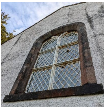
One of the broken windows.
